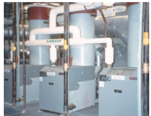
Figure 1 – High-Efficiency Condensing Boilers
